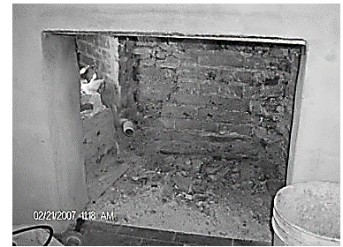
Badly Deteriorated Firebox
