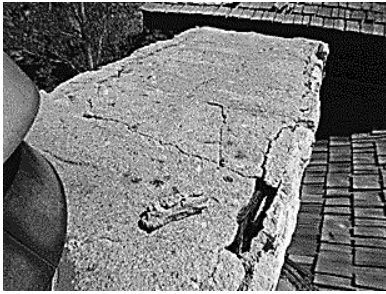
Damaged Chimney Cap
